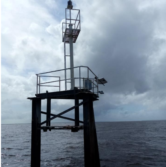
Image 1: OTT RLS Radar Level Sensor
